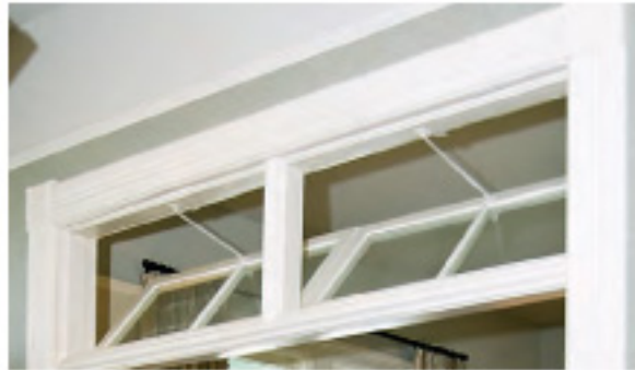
The transoms on the interior doorways were sagging before Bob Fleming was able to repair and restore them.
